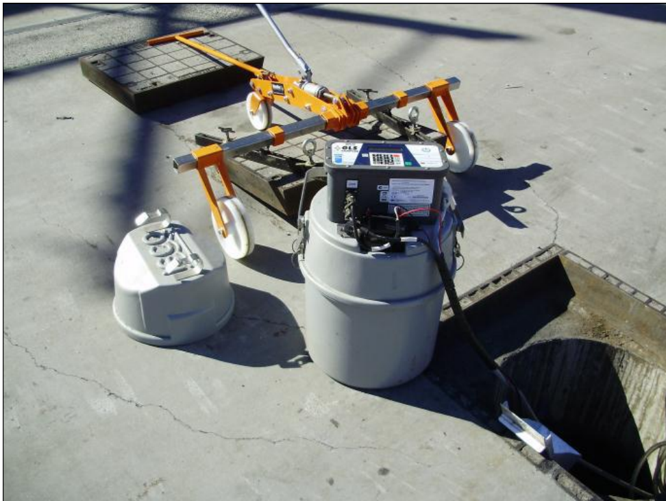
Photograph 3: Automated Water Sampler on M4 Berth
